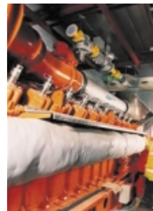
CHP plant at Royston
